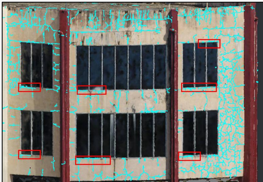
Figure 8: Detection output for the horizontal configuration at 10m. The model incorrectly identified window frames and façade elements as cracks due to high image resolution and the presence of texture-rich surfaces
