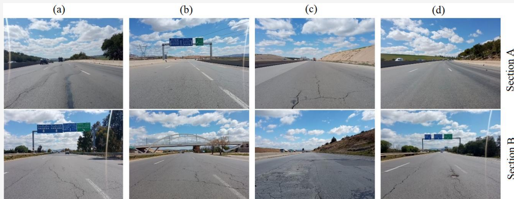
Figure 4: Principal types of defects affecting the studied sections (a) longitudinal cracks (b) transverse cracks (c) alligator cracking (d) rutting and pothole
