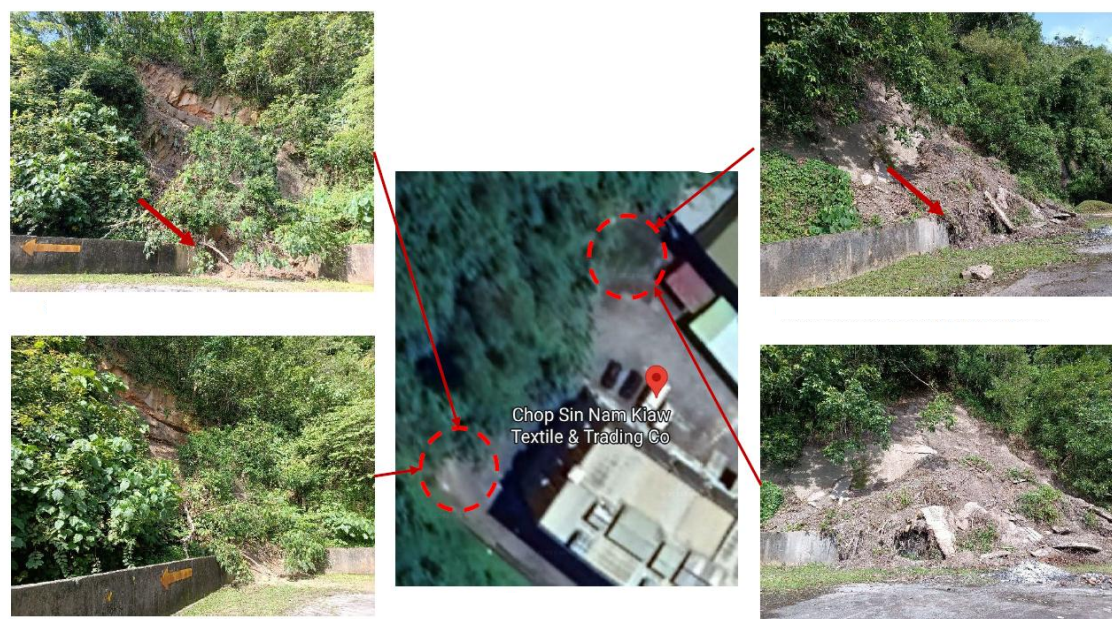
Figure 3: Landslide occurrence near a commercial building at Jalan Tutong of Kampong Madewa, Mukim Kilanas, Brunei Muara [10]
